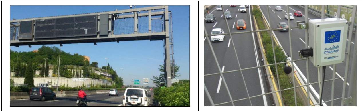
Fig. 1 – Portals carrying Variable Message Panels (VMP) with the installed sensor.
